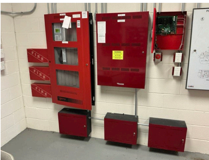
29 - FIRE ALARM PANEL
