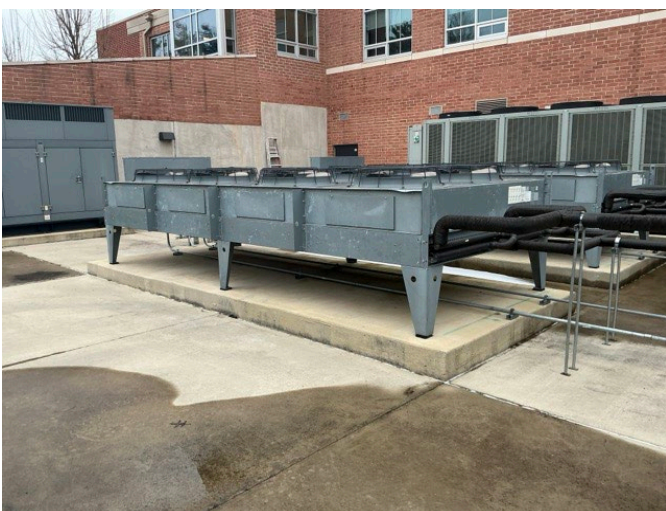
23 - COMPUTER ROOM AC UNITS
