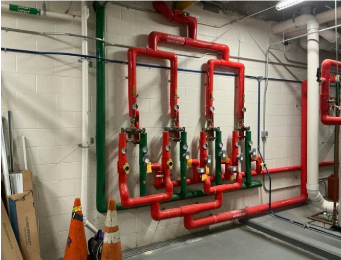
7 - PLUMBING SYSTEM PIPING
