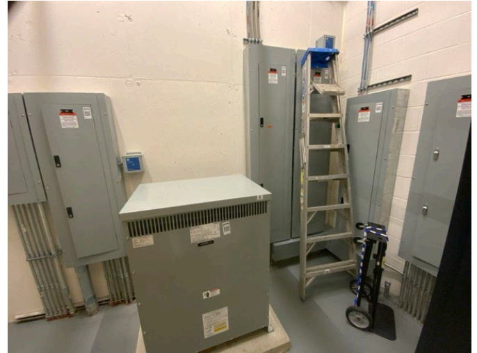
26 - TYPICAL ELECTRICAL ROOM
