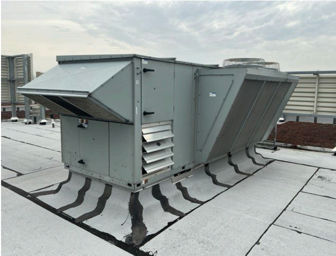
25 - TYPICAL PACKAGED UNIT
