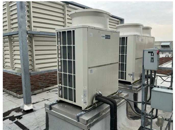
22 - VRF HEAT PUMPS
